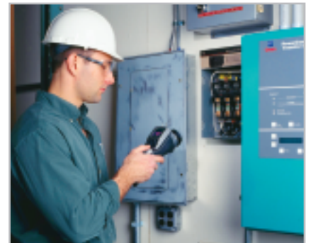
Infrared can accurately and quickly locate faults before failures, shutdowns, or even fires occur.
